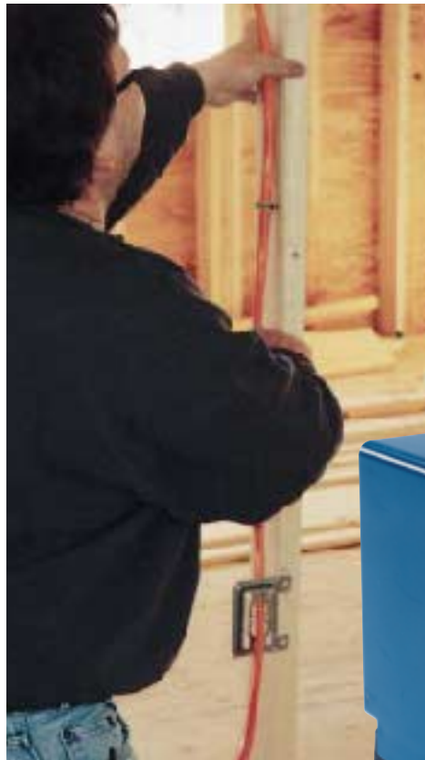
Figure 8. Avoid wiring runs in insulated walls; if you can't, run the wire in a conduit to facilitate future pulls, and use a backless electrical box. On interior partitions, all you need is a plaster ring.
