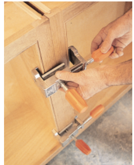
Figure 7. Pony "Cabinet Claws" are the newest weapon in the author's installation arsenal. They draw the cabinets together and keep the face frames perfectly flush at the same time, acting like an extra pair of hands.
