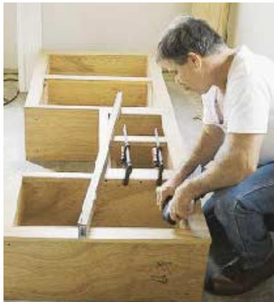
Figure 3. The author assembles the upper cabinets on the floor as a unit, shimming from the back until the fronts are straight and flush. Note the level used as a straightedge.
