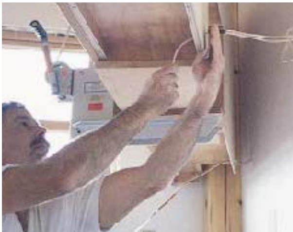
Figure 5. Wires for under-cabinet lights are roughed in at a safe height behind the wall cabinets. The author then slices the drywall to bring the wire down to the correct height at the bottom of the cabinet.
