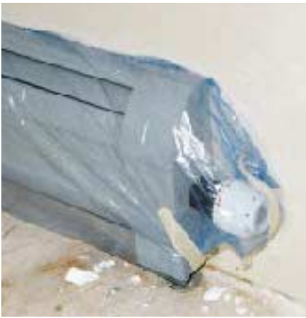
Figure 3. Thermostatic radiator valves (TRVs) allow adjustment of individual baseboards in a series loop. The plastic wrap is to protect against splatters from drywall mud.
