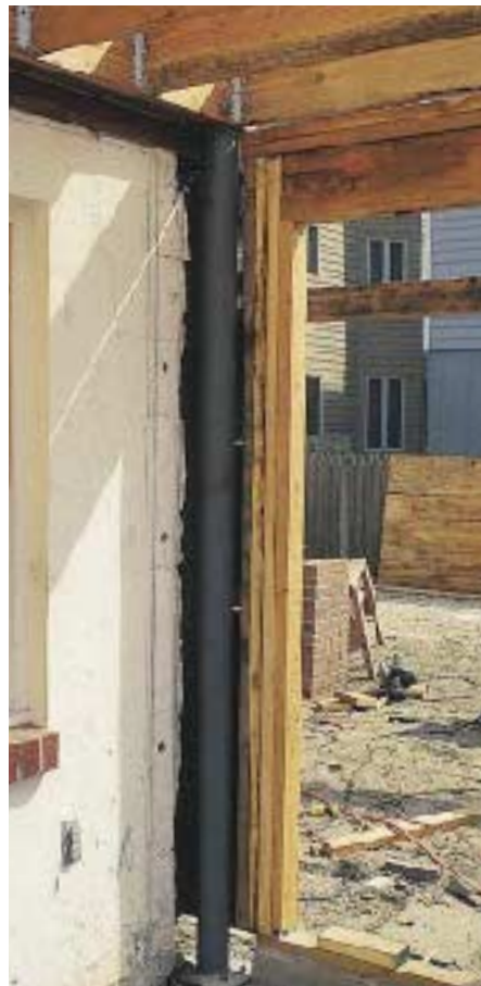
Figure 5. Once the flitch beam was bolted together, the support column was installed. Note the nonshrink grout at the bottom, used to fill the gap between the base plate and the concrete.
