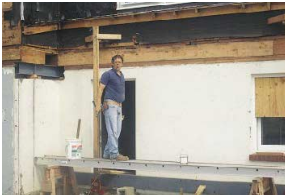
Figure 3. A new rim joist was installed to receive the first steel plates, seen here resting on the pump jacks.
