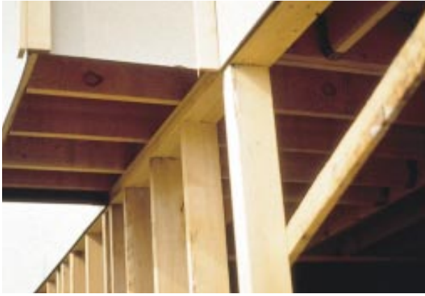
Figure 2. The floor framing in this photo, which was cantilevered to allow for a zero-clearance fireplace, follows the 1-out/2-in rule of thumb for non-bearing cantilevers. The weight of all the framing and finish materials, however, plus the fireplace and chimney, adds up to well over 1,500 pounds. The illustration shows how the cantilever should have been framed. The solution, however, depends on the species of lumber used. The author recommends that an engineer design any loadbearing cantilevers.
