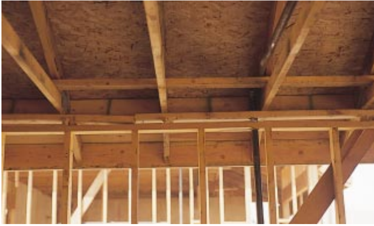
Figure 4. To correct a wavy foundation wall, the framers drove wedges between the top plates, effectively breaking the connection (photo). The best solution would have been to wedge between the bottom plate and sill, then tie the connection together with metal straps or plates, or with well-nailed, continuous sheathing (top illustration). The in-place wall can also be corrected with metal twist ties that connect the trusses directly to the studs, and with metal straps that tie both top plates to the studs (bottom illustration).
