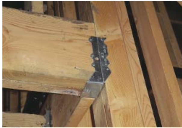
Figure 1. Bending joist hangers to conform to the framing (photo) weakens the metal and reduces the load the hanger can carry. The illustration below shows how this floor could have been framed without having to reshape the hanger.
