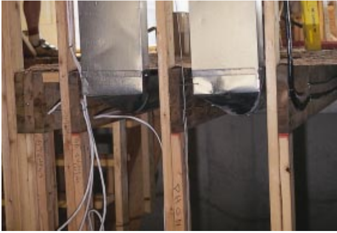
Figure 3. The missing fire blocking and edge blocking in this photo can easily be installed at the top and bottom of joists in the bays without ductwork (top illustration). Where ducts get in the way, install a metal collar, which will choke off a fire and prevent it from spreading into the wall. Where soffits above kitchen wall cabinets are framed before drywall is installed (lower illustration), the joint between the wall and ceiling also needs fire blocking.
