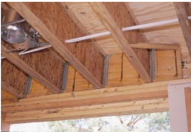
Figure 6. When there is not enough room for a conventional header, the rim joist can be doubled to take the load. Use joist hangers on 2x4 walls, where the doubled rim joist doesn't leave enough bearing surface. Also, be sure that the inner rim joist is long enough to bear on the doubled king studs; otherwise, the plate may crush.
