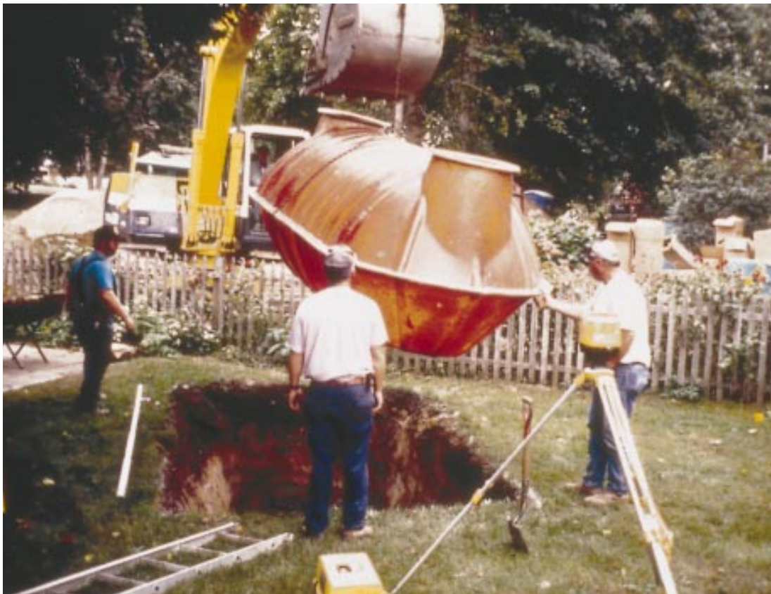
A 1,500-gallon fiberglass septic tank is lowered into position. The risers at each end will have tight-fitting covers flush with finished grade to allow for inspection and maintenance.
