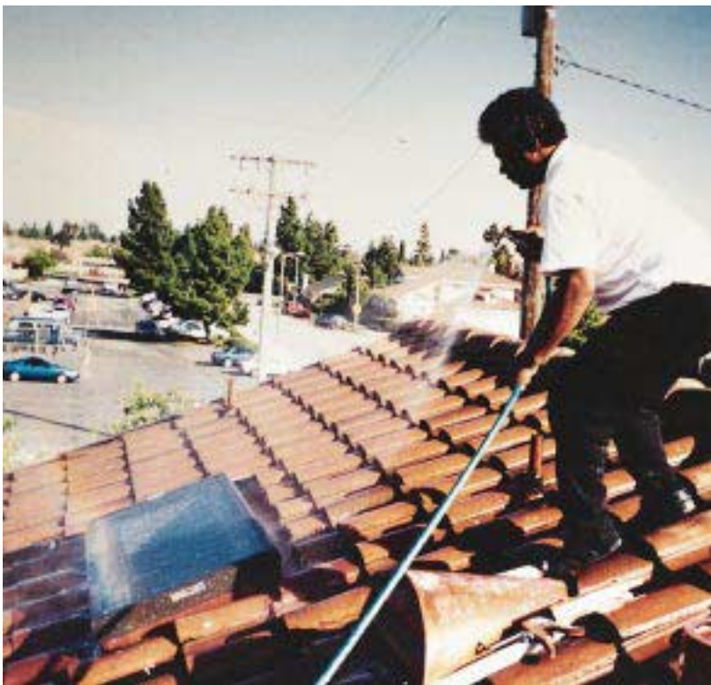
Figure 4. Before installing drywall in the skylight shaft, the author uses a garden hose to perform a leak test. The sealants he uses to repair any leaks can be applied while the roof is still wet.
