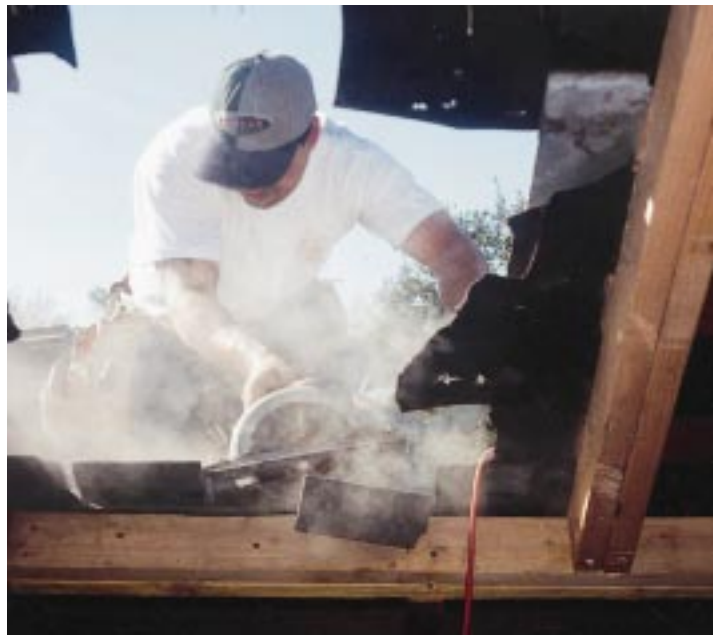
Figure 2. The skylight opening is transferred to the roof by driving nails up through the sheathing (top). The carpenter first cuts a small "breather hole" to provide light and ventilation in the attic. After framing the opening, he cuts the full-size hole (above).
