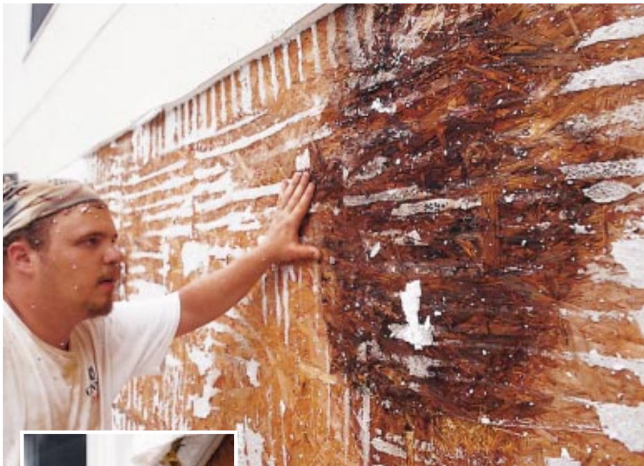
Figure 2. This three-year-old Greensboro, N.C., home was damaged when water leaks around windows and poorly-flashed roof-wall connections became trapped behind the EIFS cladding (above). Even window trim, jambs, and sills were rotted (inset) and had to be replaced.
