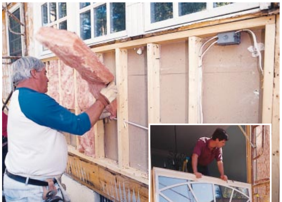
Figure 5. Hidden damage to the structure was discovered during tear-off on the south wall. The wall had to be torn out and replaced, including wiring and insulation (left), and doors and windows (right).
