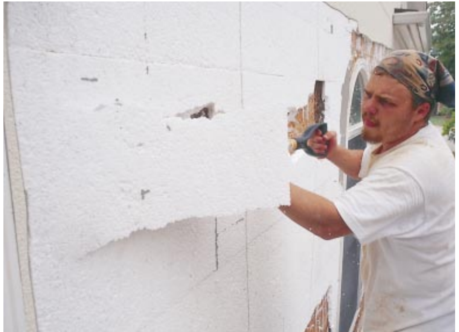
Figure 4. Large sections of foam are pried off with flat-faced shovels; smaller pieces and detailing are removed with spatulas or trowels. A crew is stationed on the ground during tear-off to clean up.
