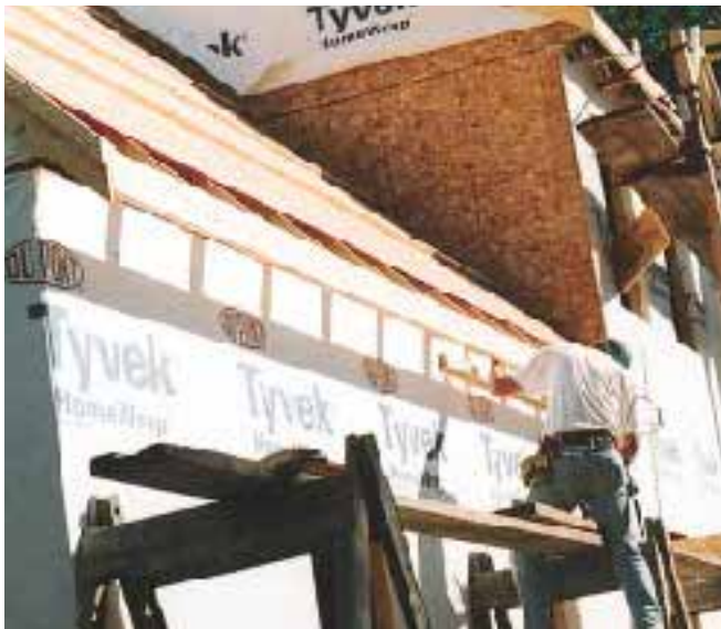
Figure 6. The authors prefer a rugged 2-by subfascia, which is installed at the truss tails before the last narrow piece of roof sheathing is filled in.
