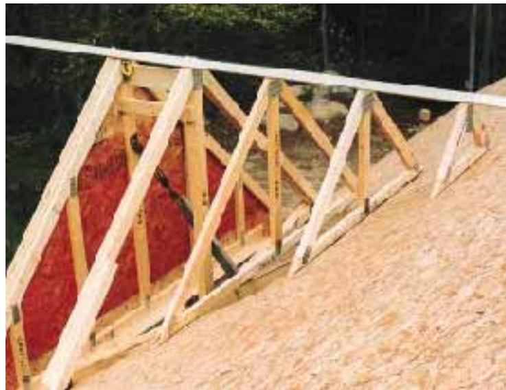
Figure 7. After the field of the roof is sheathed, the crew installs the valley kit for a small gable bumpout, leaving a gap in the sheathing below to allow for ventilation.
