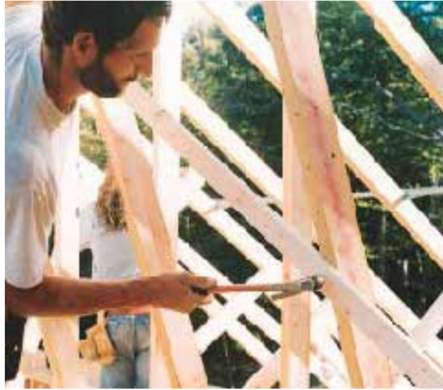
Figure 4. Temporary diagonal braces along inner webs, along with Truslock spacers on the top chords, keep the trusses from collapsing until the sheathing is installed.
