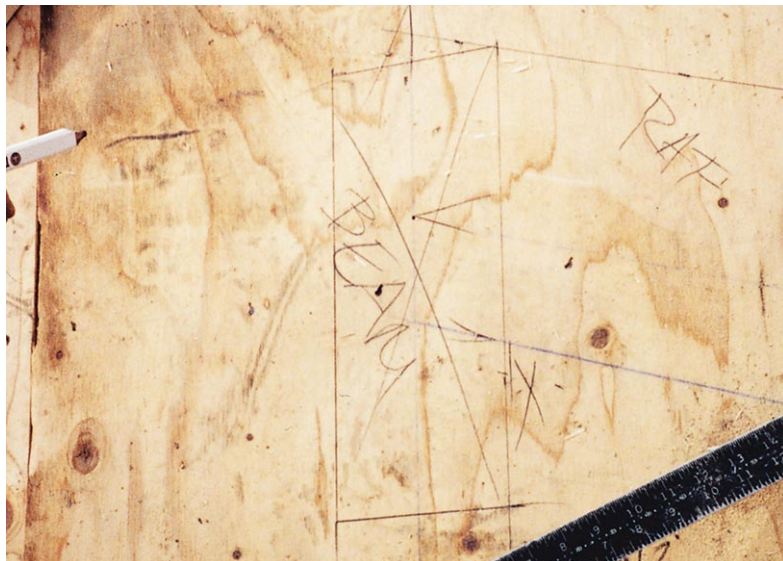
Figure 1. While laying out rake walls, the author draws details at full scale on the subfloor. To avoid having to continually refer to the plans while framing, he also writes dimensions for plates, studs, jacks, trimmers, and headers directly on the deck.
