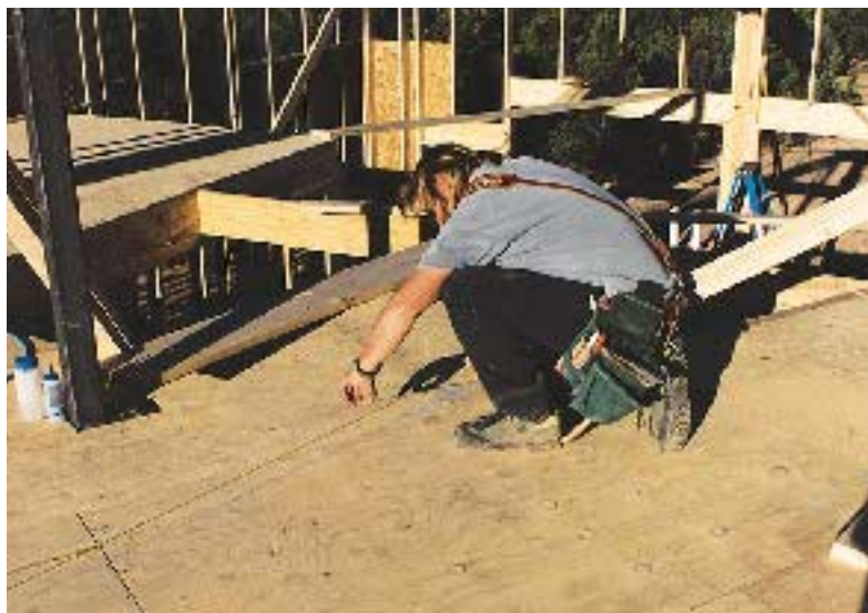
Figure 2. The perimeter of a rake wall is snapped out on the subfloor, along with lines for all studs, and headers and sills for window and door openings.
