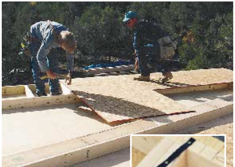
Figure 3. Framing begins by toe-nailing the sole plate to the deck (top). Before sheathing the wall (above), fasten steel binding straps around the plate and nail them to the joists. This will keep the wall from kicking out when you stand it up.
