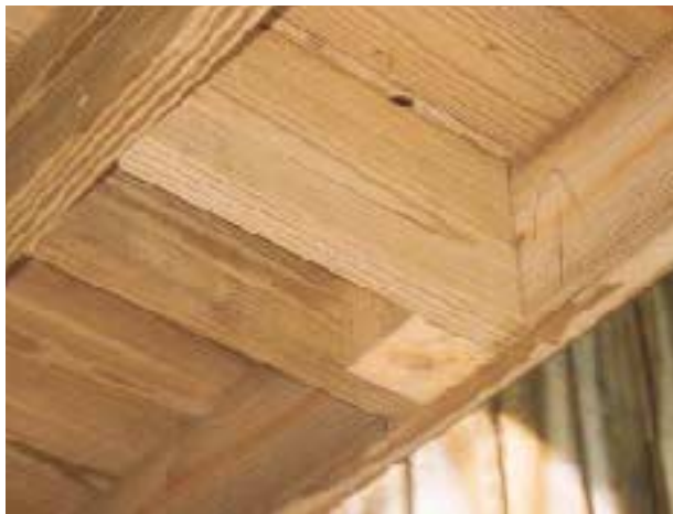
Figure 5. Secure blocking below the deck provides a snug corner for bolting the bottom of rail posts.
