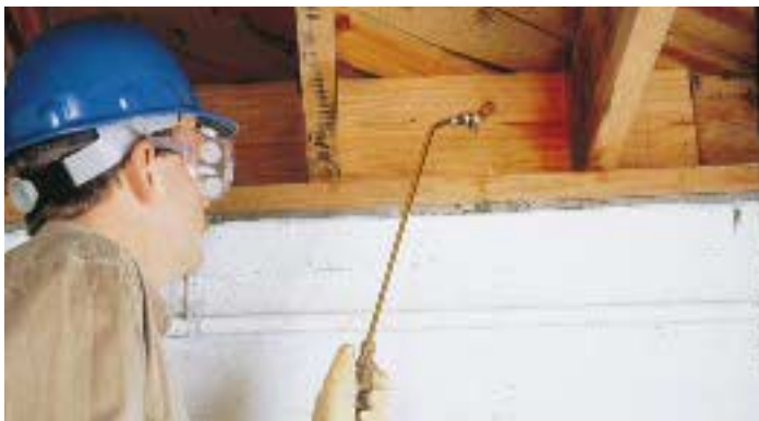
Figure 2. Areas prone to termite entry that can only be treated from one side — such as this band joist — should get two borate applications.
