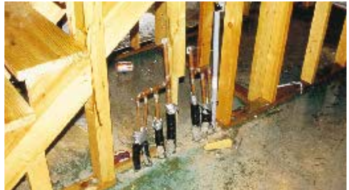
Figure 3. Borate treatment of the wood near utility pipes provides extra protection. Traditional soil treatments are also advised around such slab penetrations.
