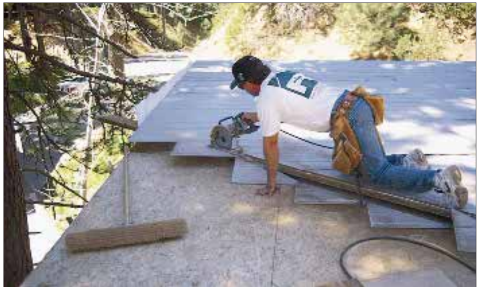
Figure 4. Aligning, fastening, and caulking the siding is a breeze when the wall is lying flat (top). As with sheathing, the author lets the siding run wild at the ends, then snaps a line along the edge and cuts off the excess (above).
