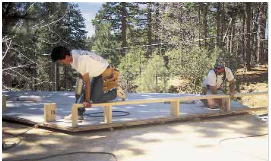
Figure 5. Before lifting the wall, the barge rafter for the rake is fastened and the rafter tail is laid out and cut in place.
