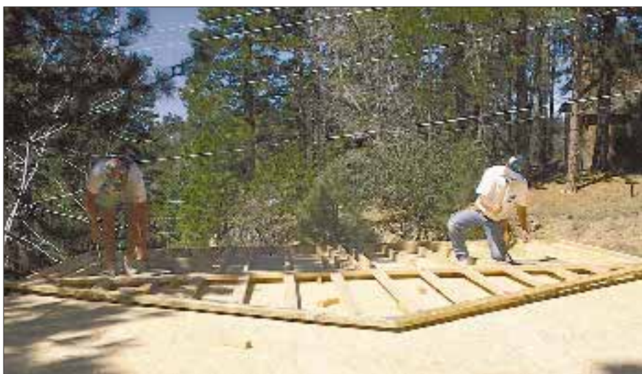
Figure 2. The author nails a gable truss to the top plate. The plan is to raise an entire second-floor gable wall, complete with windows, siding, and rake trim.
