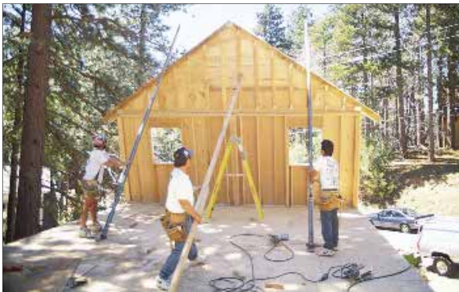
Figure 6. The author and another carpenter use wall jacks to slowly raise the heavy wall (top). Jacks must be placed to bear over a floor joist so they don't punch through the plywood. As the wall moves toward the vertical (above), permanent braces are nailed to the studs. The wall jacks can be removed after the wall plate is nailed off and the wall is securely braced to the floor.
