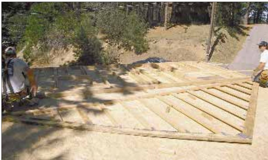
Figure 1. Since the finished wall can't be racked after siding is applied, it's crucial to check diagonals to square the wall. When the wall is raised on a level deck, it will stand plumb.
