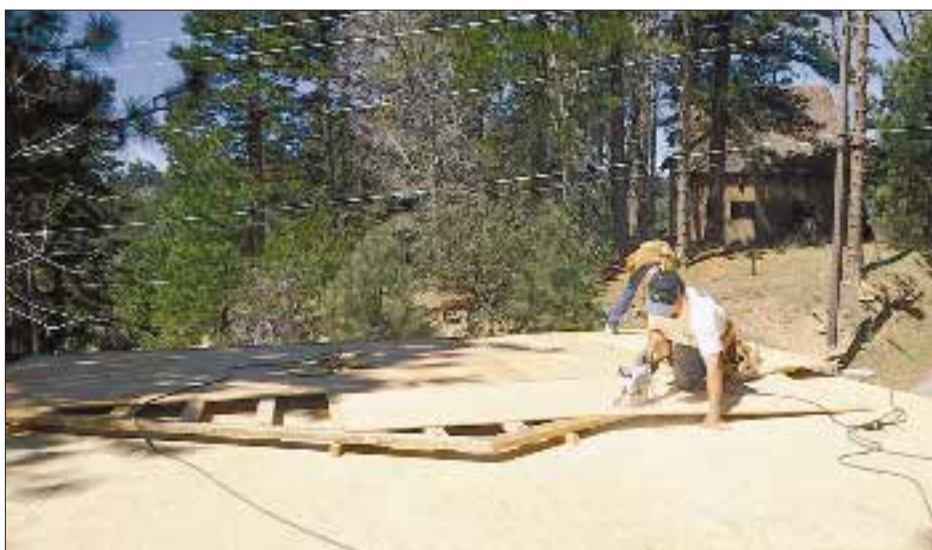
Figure 3. Applying shear-panel sheathing moves quickly when the wall is lying on the deck. Instead of pulling dimensions or figuring angles, the plywood is simply nailed in place and the excess cut off.
