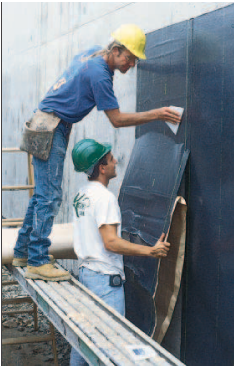
A two-person team can make good time with a self-adhering sheet membrane. One man smooths the sheet into place while the other peels away the paper.
