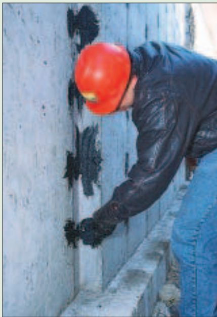
Sealing form-tie penetrations is required for some waterproofing systems. Use a grout or mastic recommended by the manufacturer.
