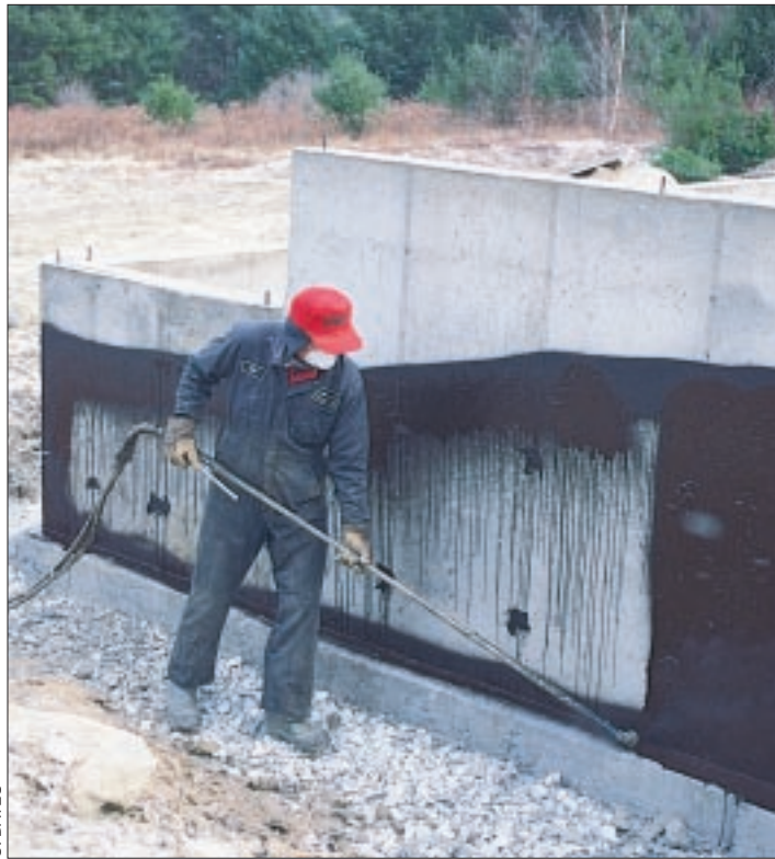
Figure 1. Liquid membranes are inexpensive and quick to apply, but it takes a skilled applicator to get the correct minimum coverage.
