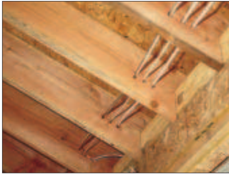
Figure 1. The rafters in the photos above are incorrectly bearing on the toe rather than the heel — risking a split in the rafter. A level cut (top) and a birdsmouth (above) are structurally the same in this respect. The wire holes in the bottom photo only make the rafters more likely to split.
