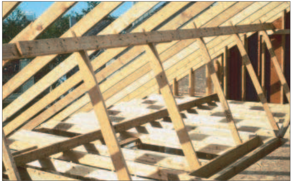
Figure 3. The rafters in this house have been stiffened with a purlin that runs the length of the roof. Because the struts that hold the purlin bear on a set of unsupported ceiling joists, however, chances are that the ceiling will eventually crack. To properly support the roof, the braces need to go from the purlin to a bearing wall.
