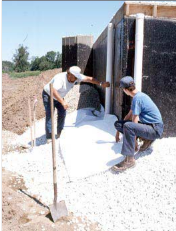
Figure 3. Before backfilling, always install a good perimeter drain, using clean stone and filter fabric to prevent the drain tile from clogging over time. Here, a foundation contractor fits the filter fabric around a vertical flush tube, which allows the drain tile to be cleaned to prevent clogging.
