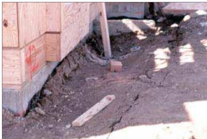
Figure 5. Settlement can occur rapidly in poorly compacted fill. Water collecting in the low spots may cause basement leakage even before the house is completed.
