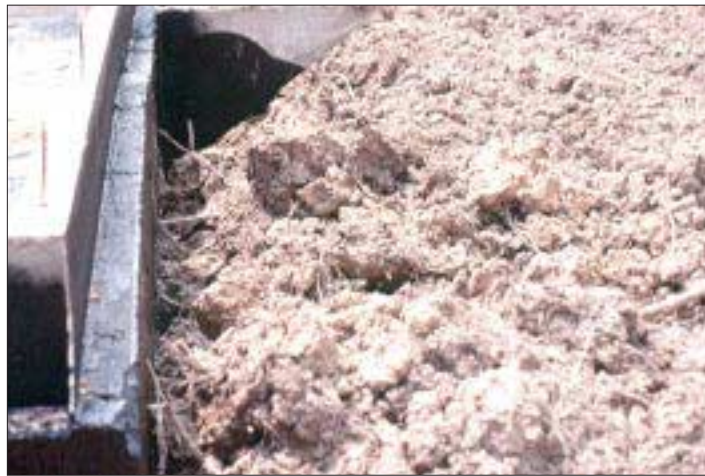
Figure 4. Backfill soil should be free of tree roots, sod, and other organic materials that make the fill porous. Such fill can't be properly compacted and is guaranteed to settle with time.
