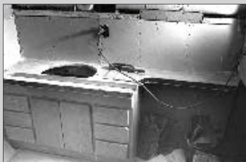
(A) In preparation for laying the tile on this vanity top, the author fastens the tile backer (Dens-Shield) over the \frac{3}{4} -inch plywood base, then attaches sink metal to the counter edge.
