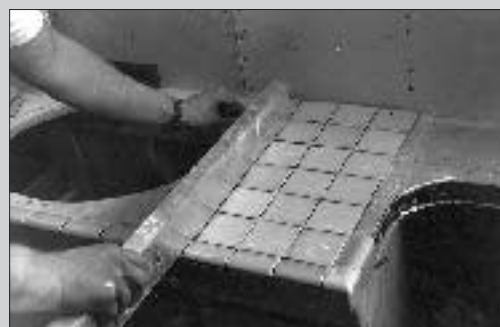
(F) He lays the field tiles in place, checking for exact alignment with a straightedge.
