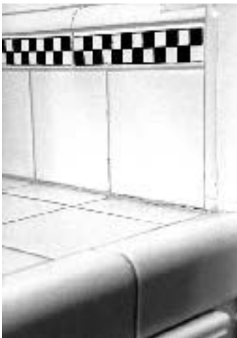
Figure 3. Critical joint. The joint between the countertop and backsplash is very susceptible to cracking because the cabinet base and the wall expand and contract at different rates with moisture and temperature changes. Instead of grout, the author recommends using a colored caulk to match the other grout lines.
