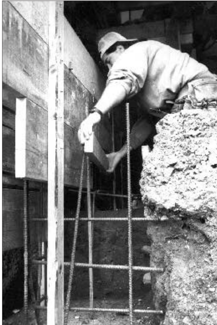
Working in tight quarters, a carpenter builds a form for a replacement foundation wall.
