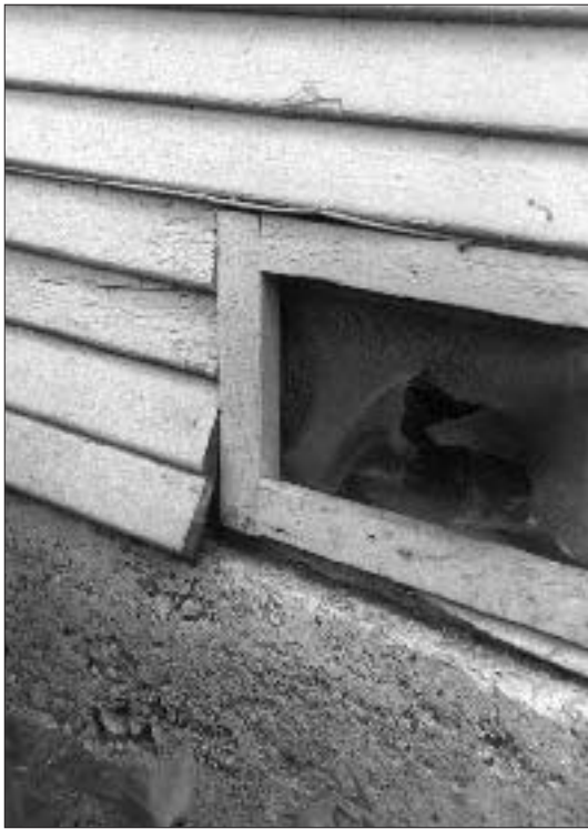
Figure 1. Signs of trouble. Unreinforced concrete foundations often fail, either from seismic activity or poor drainage. Hydrostatic pressure has caused this stemwall foundation (left) to tilt outward, pushing out the bottom courses of siding. This grade beam (below) has separated into sections, possibly as the result of earthquake. The damage in both cases is beyond repair; the foundation sections must be replaced.
