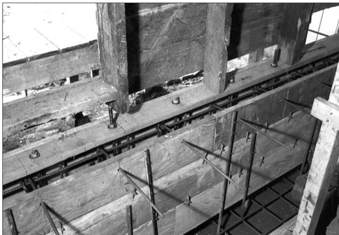
Figure 5. Preset anchors. While forming the new foundation, the author secures the new mudsill to the wall framing, then suspends anchor bolts and hold-downs as needed. The space between the mudsill and the form allows room for the concrete pump hose during the pour.
