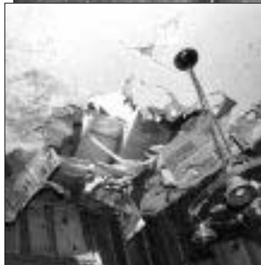
This house in South St. Paul, Minn., was destroyed by a ruptured water heater (inset right) that blasted its way through joists and rafters (inset left) before coming to rest in a neighbor's yard.
