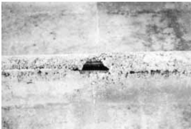
Figure 1. Honeycombing can be caused by poorly compacting fresh concrete or by large aggregate getting stuck between the reinforcement. To prevent the latter, the coarse aggregate should be much smaller than the smallest space between the reinforcement.
