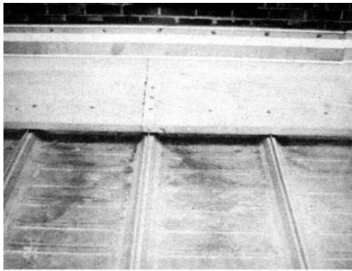
Figure 3. The stains and corrosion on these aluminum-coated panels are the result of wet mortar that spilled while repointing the end wall. Care should have been taken to protect the panels with plywood or tarps. Dry mortar, however, poses no threat.
