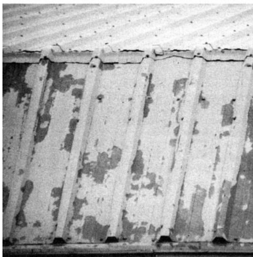
Figure 4. A field-applied paint, such as the coating on this metal roof, can be expected to last only five to seven years. High-quality factory-coated panels, however, can last over 20 years.
