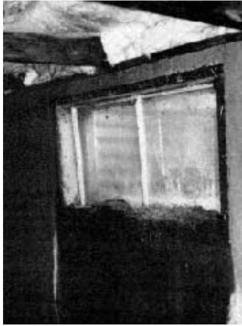
Plastic sheeting on a crawlspace floor doesn't help when it's under water. The results: rotted 2x12s, a rusty window frame, and moss growing in the window sill.
