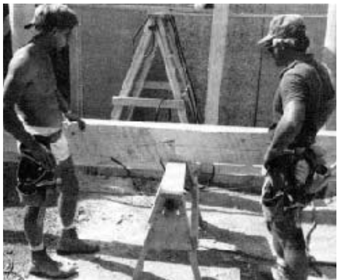
Small crews should think through risky operations, like raising this scarf-jointed beam, with safety in mind. The crew leader needs to set the tone.
