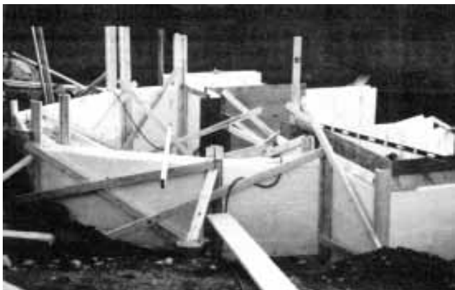
Figure 4. The bracing required for the foam forms is considerably less than for conventional concrete forms. Here, the author supported the foam forms with vertical 2x4s every 5 feet, braced back to the ledge, with diagonal 2x4 cross bracing in between.
