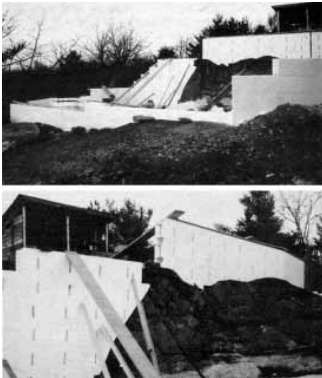
Figure 3. Since the author was building over solid granite, he chose not to use a spread footing, but to scribe the blocks directly to the ledge. The planks are temporary supports to keep the unfinished form from blowing over. The close-up view shows the wooden nailers on the inside face for drywall.
