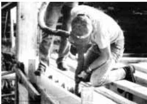
Figure 1. To prevent rupturing or dislodging the foam foundation blocks, a builder uses a 2-inch hose from a pump truck to shoot concrete straight down into the core.
