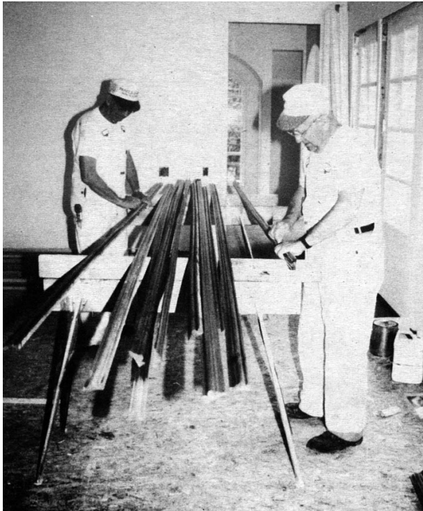
Many painters prefer to sand, stain, and prevarnish the trim before installation. The final varnish coat goes on with the trim in place.
