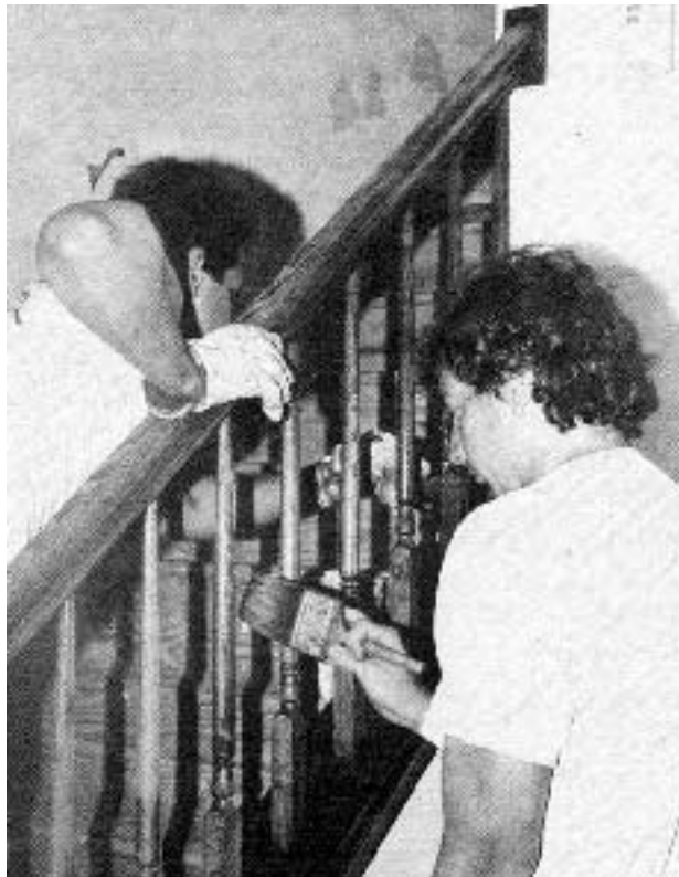
Painters apply the finish varnish coat to stained oak. For best results, they need a dust-free work place.
