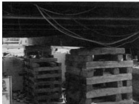
Figure 2. Stacked like Lincoln logs, squares of cribbing support I-beams, which support the house.
