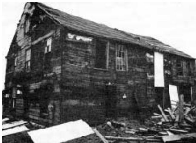
Cooper's crew prepares to dismantle the 1660 Park Homestead. The house's individual pieces are numbered and lettered so the crew can reconstruct the house exactly as it stands now.
