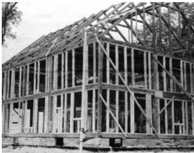
The Park Homestead is here being reconstructed in Shelter Island, N.Y. Cooper has added new framing members between the original timbers as part of the overall effort to upgrade the house to code.
