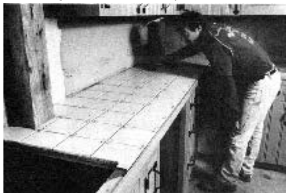
Figure 1. Check the glaze hardness before choosing an Italian tile. On counter tops, the hardness should rank in Group III or IV. This tile is set on Durock backer board and uses a strip of wood edging.
