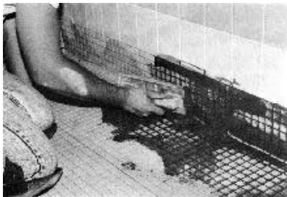
Figure 7. Apply the grout with a rubber float, and work in an area no larger than 20 square feet at a time.
