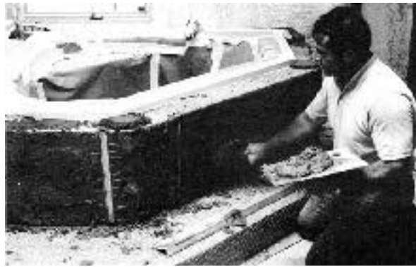
Figure 3. With thick-set mortar, you can level or plumb uneven framing and contour the mortar bed to any angle. Mortar is applied over wire or mesh lath.
