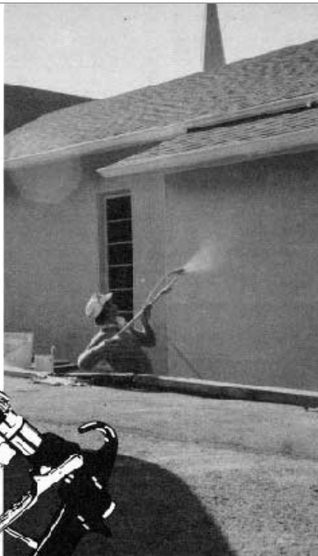
Spraying with airless spray guns can bring tremendous labor savings to large exterior jobs. But some surfaces such as stucco often call for prep coats applied with brush and roller.
