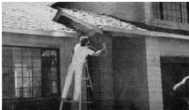
Figure 1. In addition to saving time, spraying can also make life easier in hard-to-reach places like the underside of this overhang.
