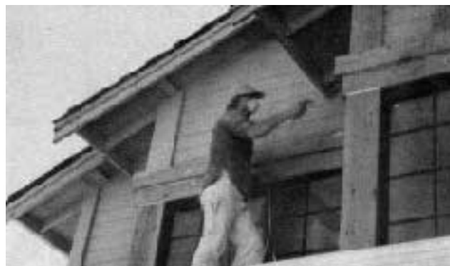
Figure 3. Eaves are typically a good choice for spraying since their smooth surfaces accept paint evenly. However, take full precautions against overspray—tarping, masking, and just plain vigilance.
