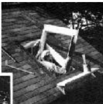
Figure 5c. Then set the skylight box or flashing in a bed of roof cement.
