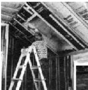
Figure 5a. This skylight fits between two 16-inch on-center rafters. After framing the opening with double headers, drive a spike in each corner to mark the opening on the roof.
