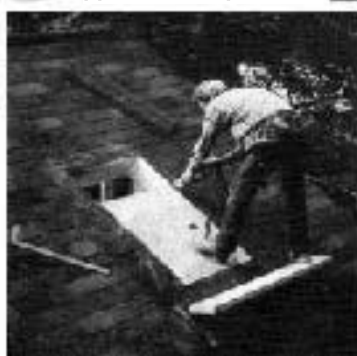
Figure 5b. After stripping the shingles, cut the opening, and seal the roofing paper to the deck with lap cement.
