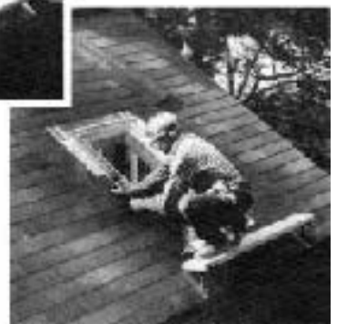
Figure 5d. Shingle it up holding shingles back 1/2-inch from the curb. Never nail through the flashing or flatten the turned edge (rain gutter) of the side flashing. For the best protection against leaks, use step flashing.
