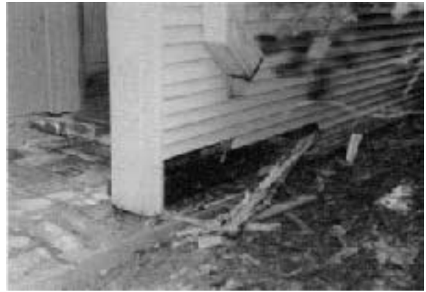
Figure 1. The siding and sill were within 2 inches of the ground in places, such as this garage wall.
