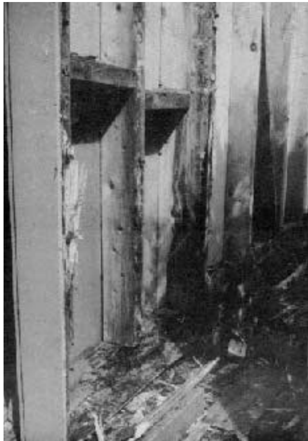
Figure 2. Damage to the garage sheathing and framing extended from grade to 6 feet up.
