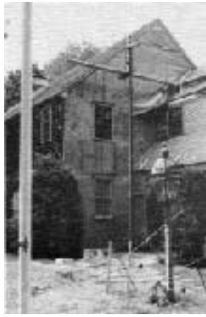
Figure 6. More than 90 percent of the sheathing had to be replaced due to moisture damage and delamination.
