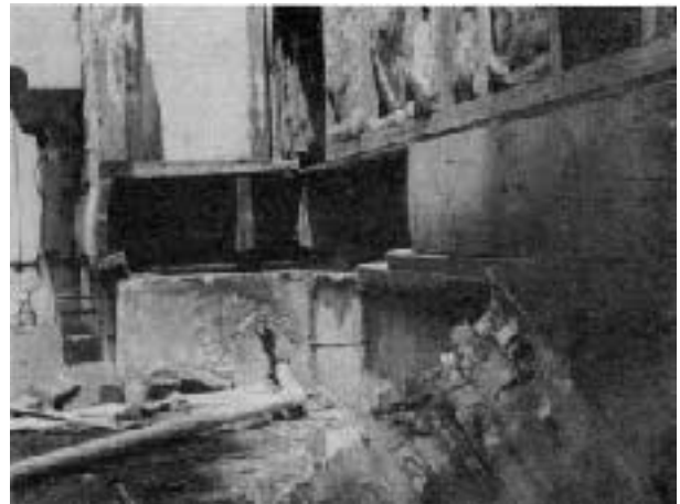
Figure 4. The double 2x4 sill was falling off the foundation due to its cantilevered placement.
