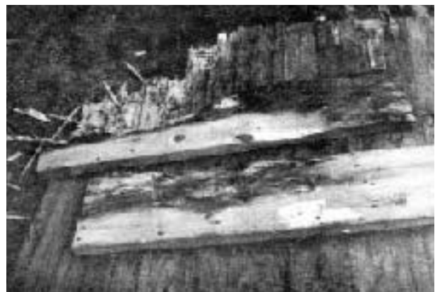
Figure 5. The second-floor band joists at the overhand suffered substantial rot.
