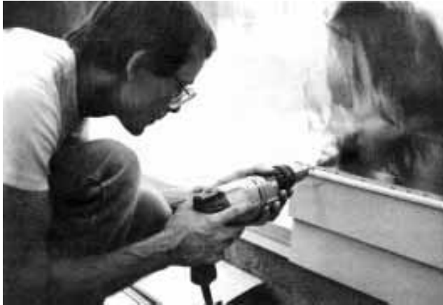
Figure 3. For roof and siding, the author chose inert materials like metal siding and metal roofing because their baked-on finishes have minimal outgassing.
