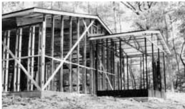
Figure 1. Steel framing members cost more than twice as much as wood, but you can save by framing 24 inches on-center and eliminating termite protection.
