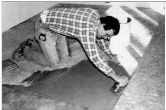
Figure 2. For floors, ceramic tile was used because it is inert. Though the tile adhesive outgasses, the tile and grout block the gas from entering the living area.
