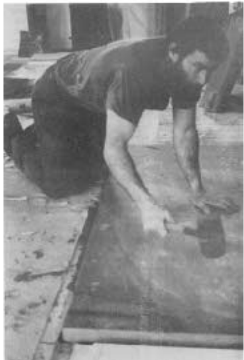
Mortar must first be worked into the lath (top). If a large stone is to be set, a straightedge can be used as a screed to prepare the mortar base (center). Once the stone is set, it must be beaten in (bottom).
