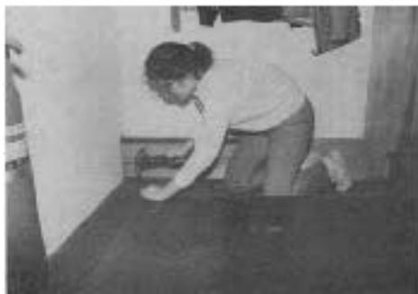
▶ Nailing Machine A power stapler would have been quicker, but advertising director Malaine Drumheller makes quick work of the hard-board facing. The other side will be covered with Homasote.
