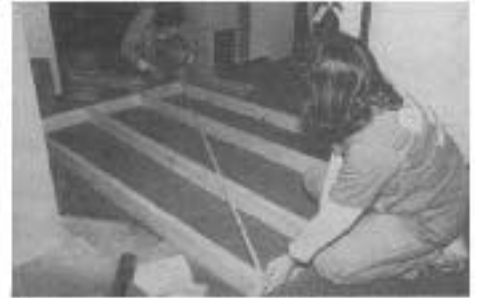
▶ Prototype The crew assembles the frame for the first 4x6-foot partition section. If this one works out, the other seven modular sections will be mass-produced.
