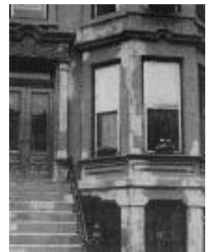
This contractor didn't do any test patches when repairing this unpainted brownstone—with spotty results.
