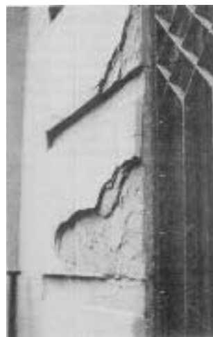
Although spalling doesn't pose an immediate structural problem, the exfoliation of bedded brownstone layers will accelerate as water enters the rough, deteriorated surfaces.
