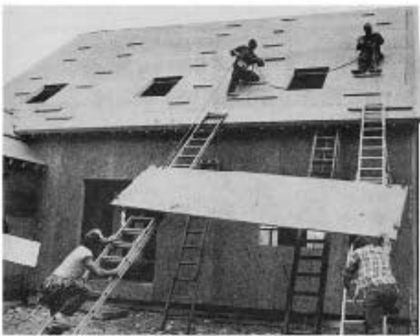
A little ingenuity can replace a crane when installing roof panels. This 4x16-foot panel is 4 1/2 inches thick and weighs in at about 250 pounds.
