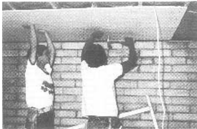
One of Aztech's three types of radiant ceilings being installed. The SunComfort panels shown here are made of 5/8" gypsum board in which radiant cables are embedded, producing a completely concealed heating system.
